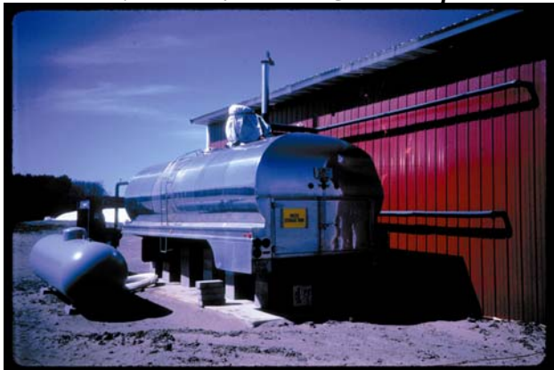
Hot Water Storage
