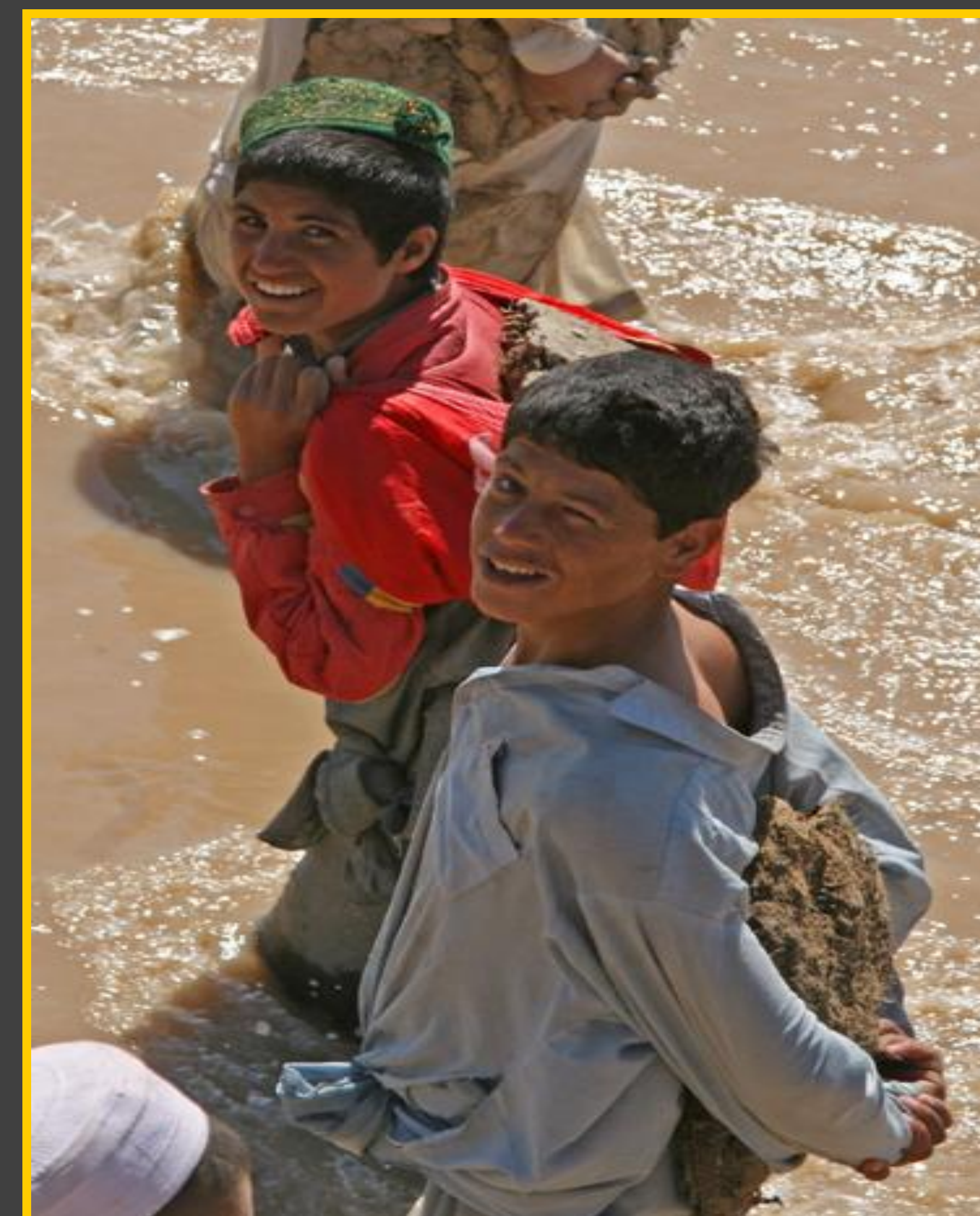
Above: Afghan villagers construct a sod diversion dam. Quality improvements can serve to limit the amount of labor necessary to operate and maintain irrigation infrastructure. (Fipps, 2006)
