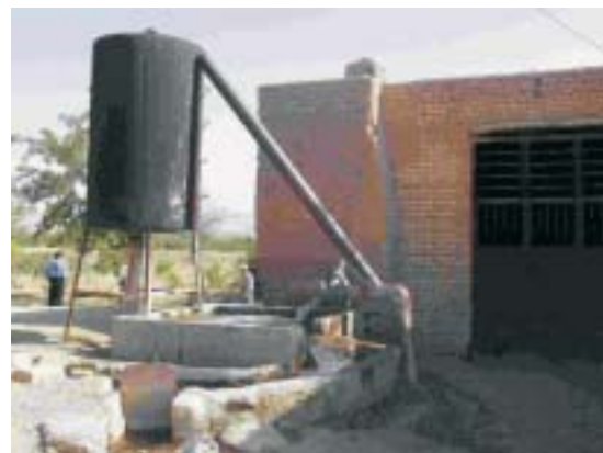
A pumping station (well)
