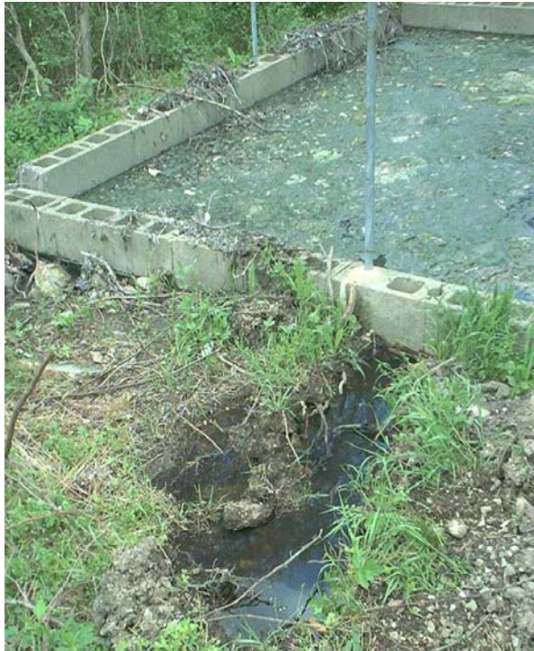
Figure 39. Failing lagoon system
