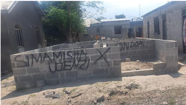
Figure 1: Construction stop order issued by the local leaders in Teta subward
