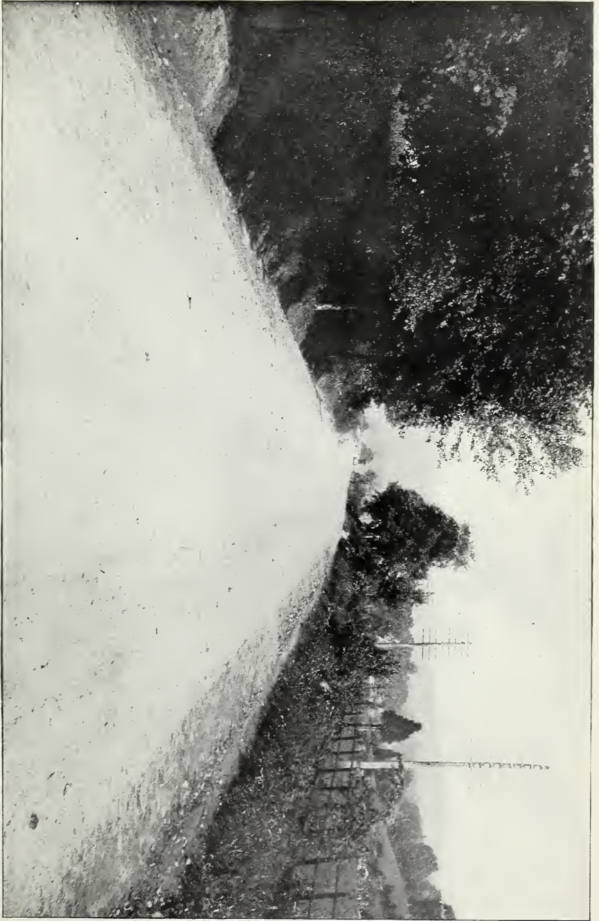
ELMSFORD AND EASTVIEW ROAD, WESTCHESTER COUNTY, N. Y., AS IN PROGRESS OF IMPROVEMENT IN 1901. Base of local gneiss; top of Rockland-Lake Hudson-River trap rock, bound with Clinton-Point Hudson-River limestone screenings.
