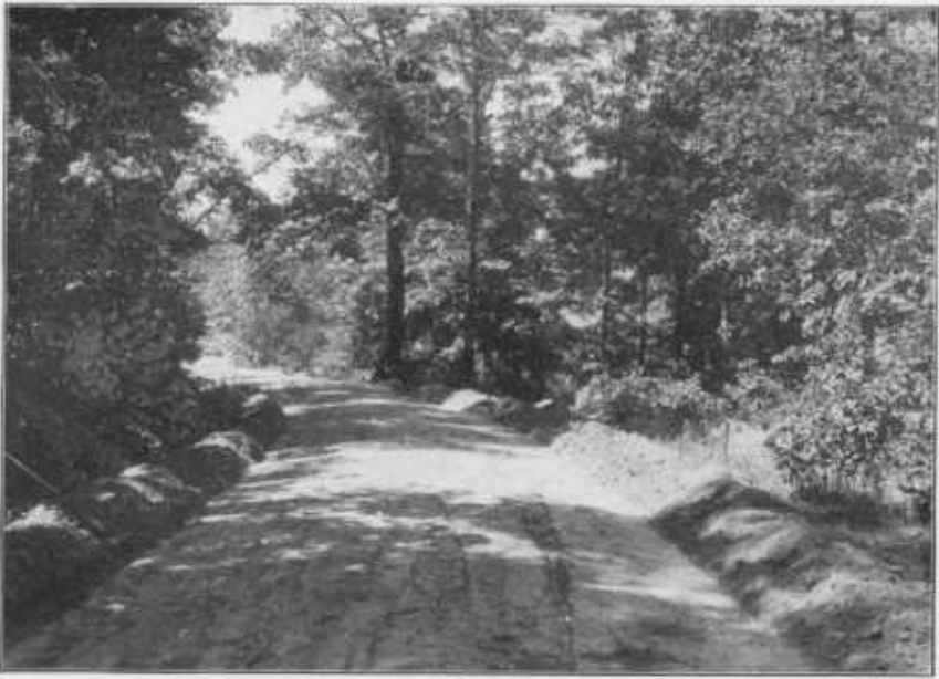
FIG. 1.—THE ROLLED FOUNDATION OF AN OBJECT-LESSON ROAD BUILT AT HOT SPRINGS, VA., UNDER THE AUSPICES OF THE OFFICE OF PUBLIC ROAD INQUIRIES OF THE DEPARTMENT OF AGRICULTURE.
