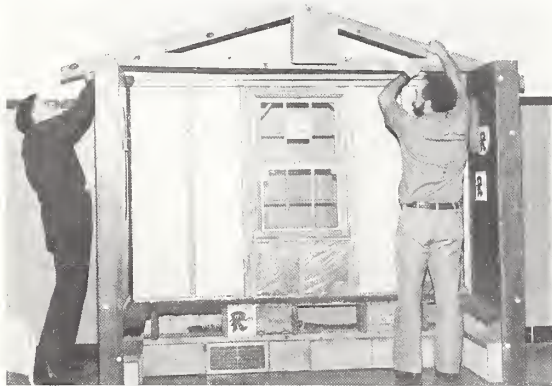
Extension workshops for builders and homeowners teach proper methods of installing insulation.
