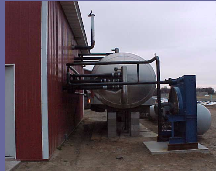
hot water storage - 180F
