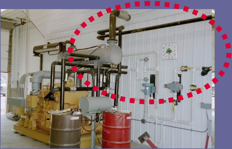
heat exhaust recovery
