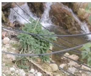
b. HDPE used to convey water from creeks
