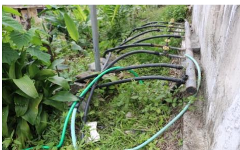
d. HDPE hoses connected from group reservoir to individual farms
