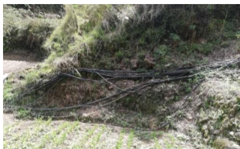
e. HDPE passing by farms need to be watched for leaks from springs to individual farms
