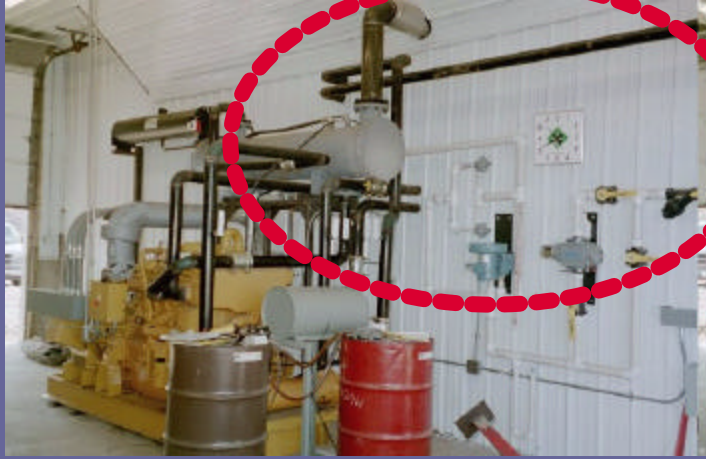
heat exhaust recovery
