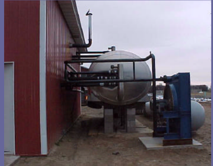
hot water storage - 180F
