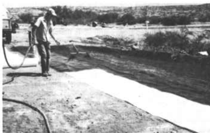
Figure 13.—Spraying asphalt emulsion base coat on fiberglass matting for a catchment treatment.
