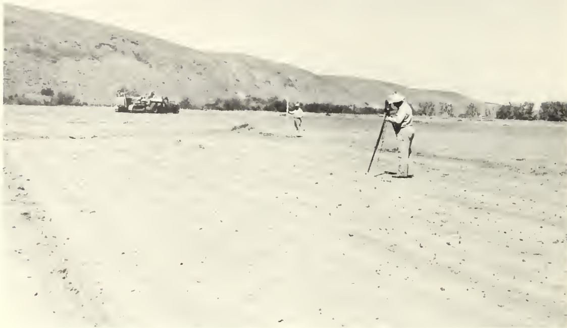
Figure 32.--Land is leveled for more efficient application of irrigation water, subbasin 3. SCS photo. 7-736-2
