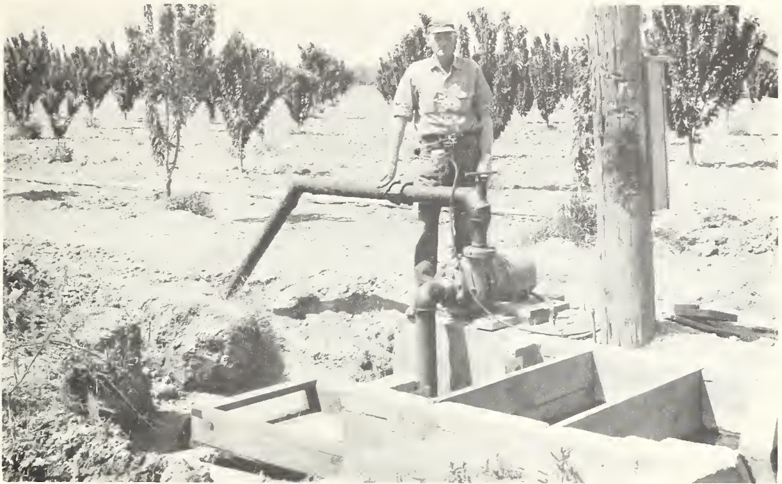
Figure 34.--This structure screens out weed seeds and some silt from irrigation water in subbasin 1. SCS photo. 7-1116-7
