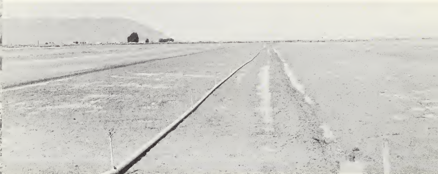
Photograph 49. - Land-leveling and the installation of sprinkler irrigation facilitate a more positive control of water. Battle Mountain Sub-Basin.
