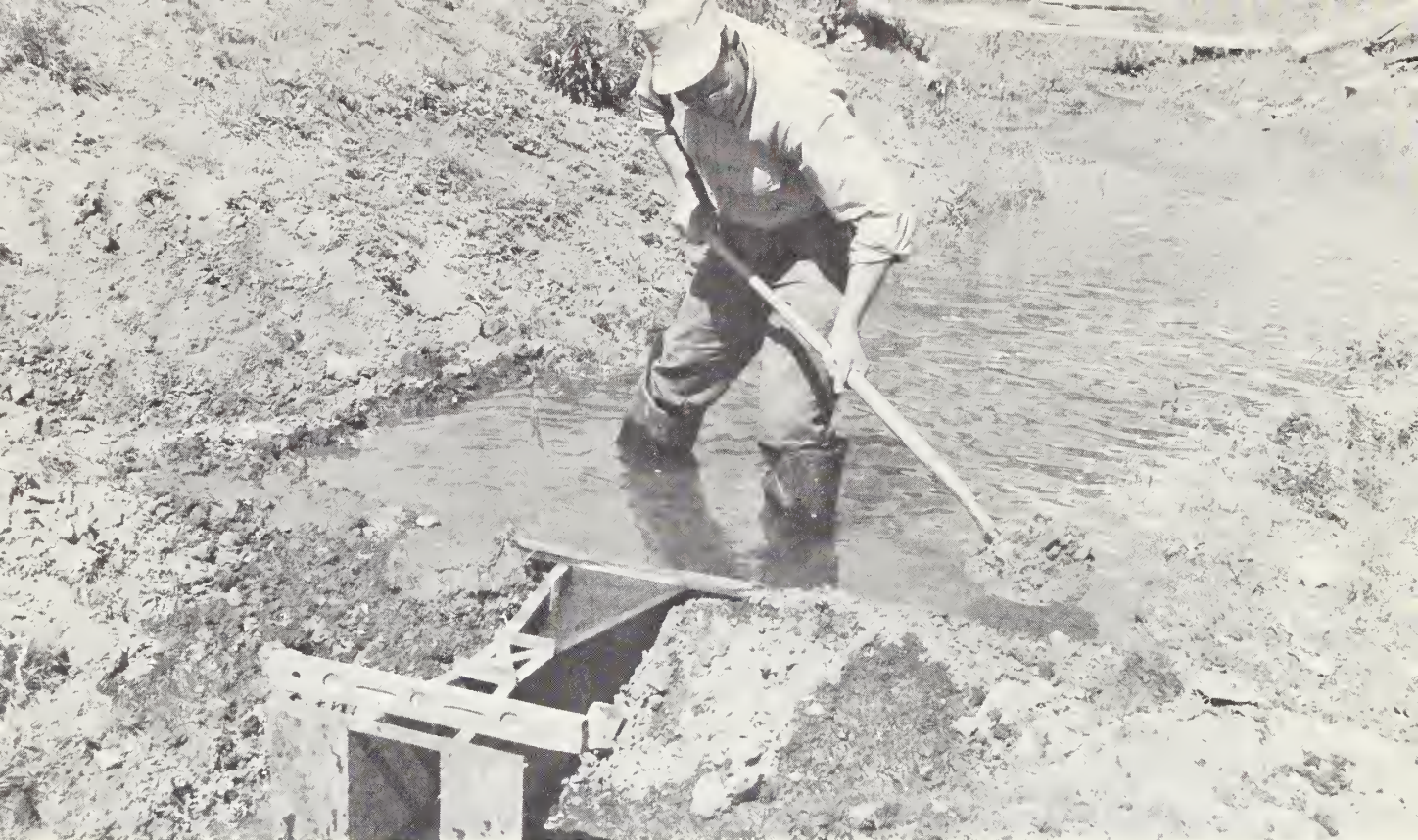
Photograph 31. - Measuring water at or near the point of use by means of a Parshall flume.
