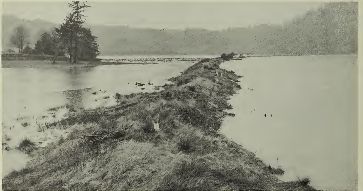
Photo 23.--Inadequate dikes and tidegates allow flooding along the Little Nestucca River in Oregon. SCS photo
