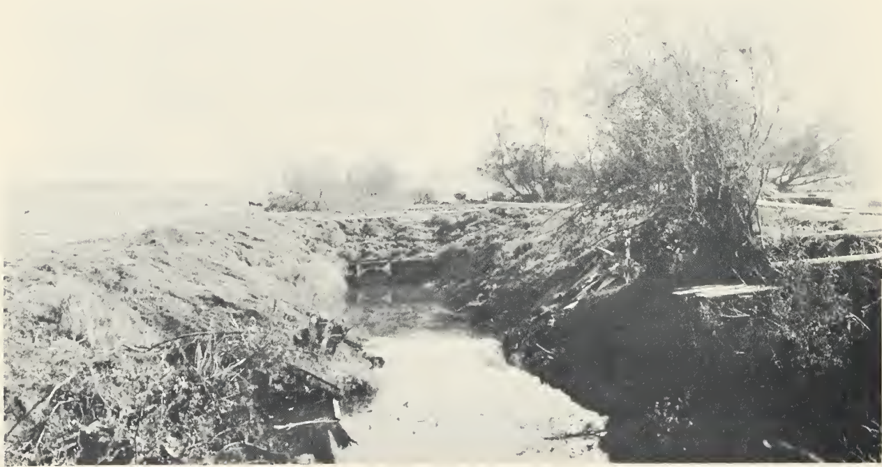
Figure 33 Automatic floodgate on Coquille River Fishtrap Drainage District near Arago, Coquille Subbasin, Oreg.
