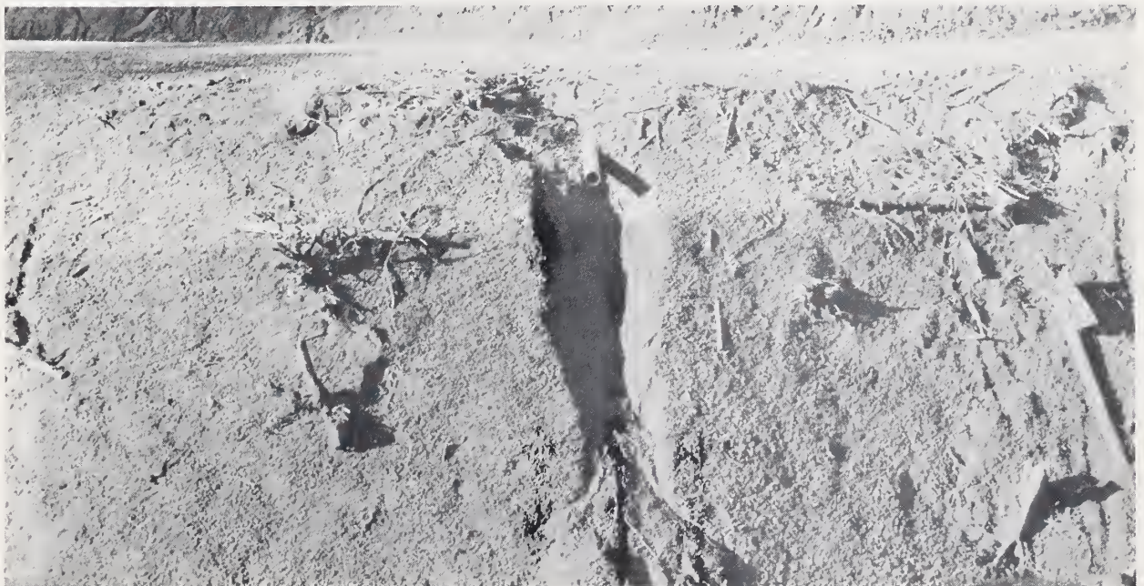
Figure 27 Improper culvert installation has resulted in soil losses on this forest road in the Coquille Subbasin, Oreg.
