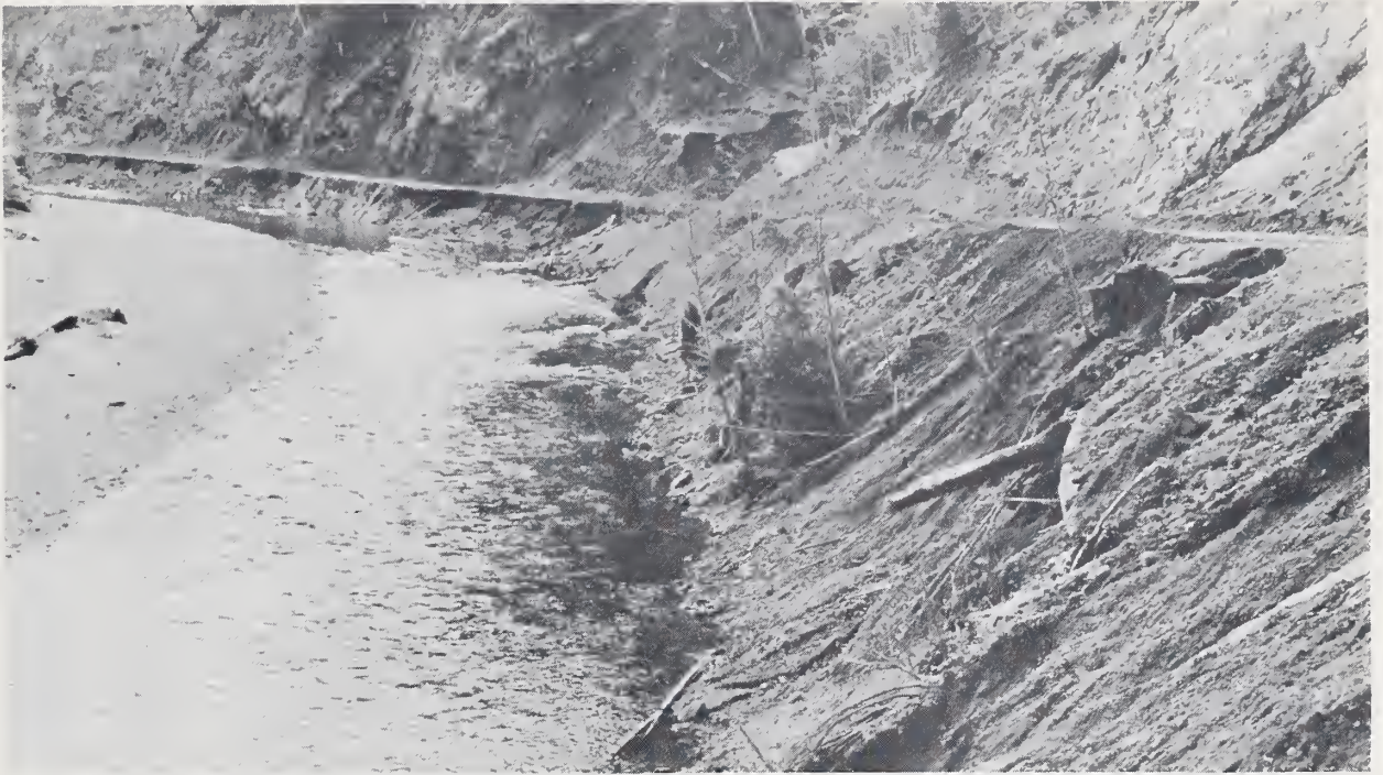
Figure 26 Improper road location and construction has resulted in excessive soil disturbance and erosion on a forest road in the Coos Subbasin.
