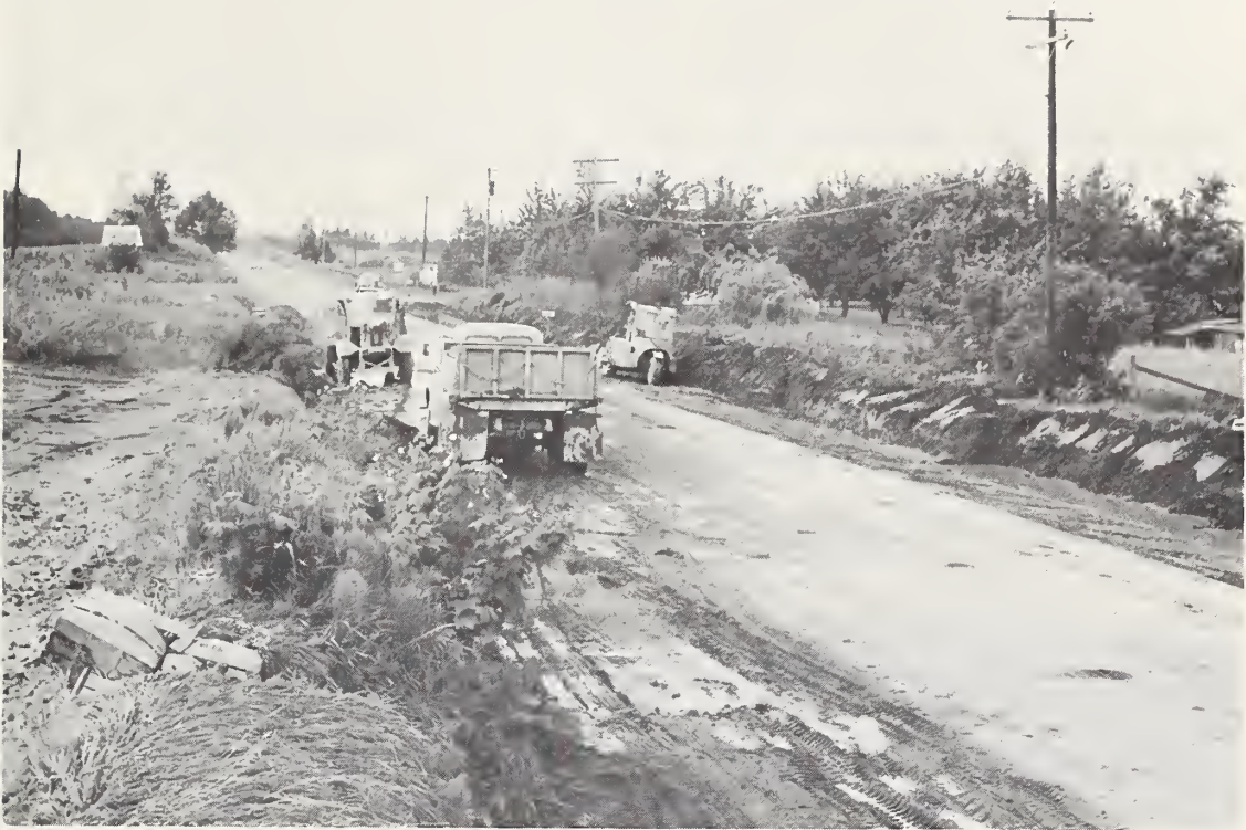
Photo 31.--A Multnomah County road crew is removing sediment from N. E. Halsey St., subbasin 11. SCS photo. F-128-8
