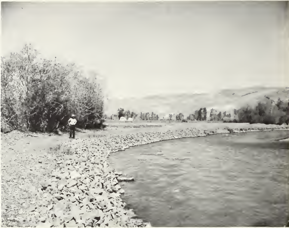
Figure 22 Bank erosion effectively controlled by rock riprap. John Day River below Dayville, Oregon.
