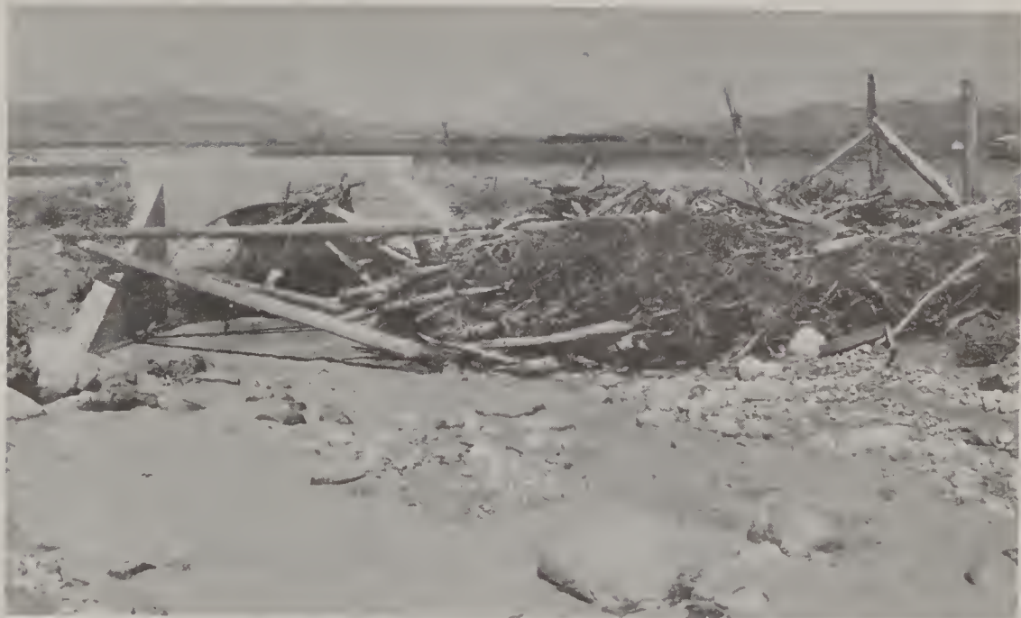
Flood damages in 1959 in the Cedar City area included channels and culverts plugged with debris (above); irrigation ditches filled with mud, and flooded cropland (below).
