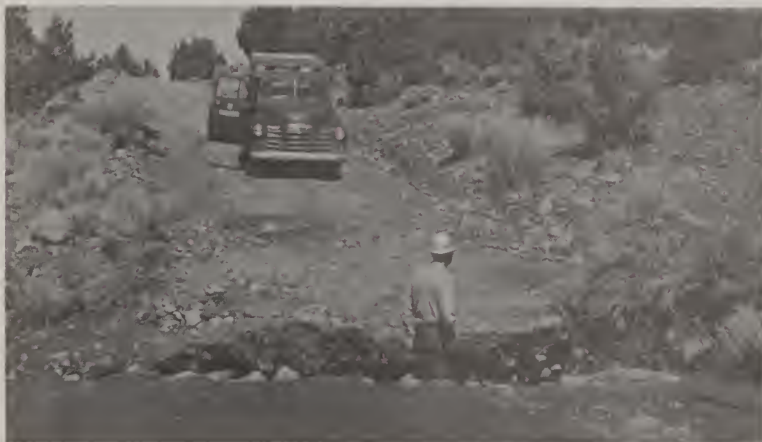
Road and bridge washed out in a flood on the South Creek Drainage, Beaver Watershed, 1959.
