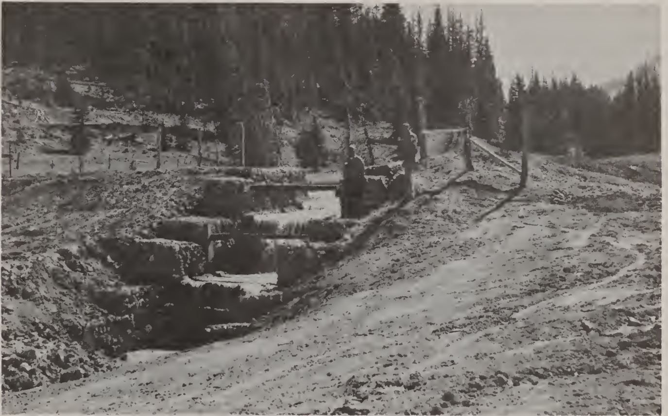
Drop structures (above) and gully plugs (below) are effective means of stabilizing streams and gullies.
