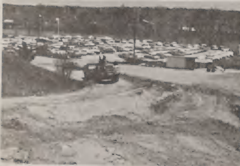
Erosion is a problem on construction sites,
