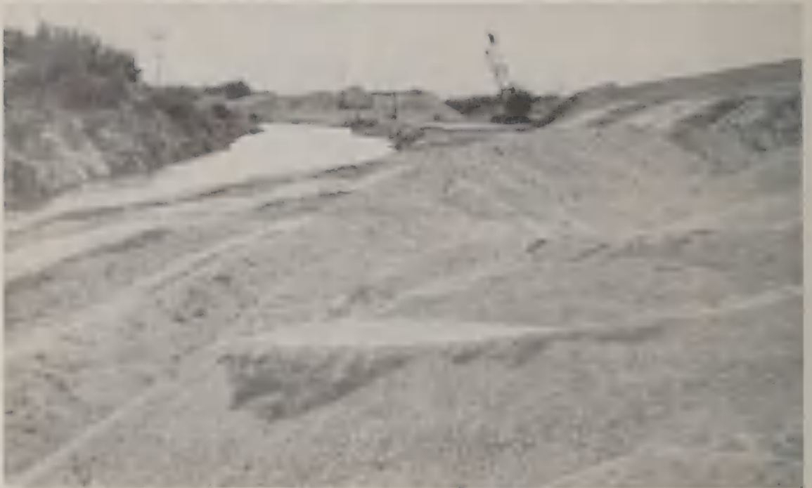
Photograph 19. Downstream along Florence-Casa Grande Canal in immediate vicinity of Ashurst-Hayden Diversion Dam. Note sediment (right) which has been dredged from canal. (SCS Photograph)
