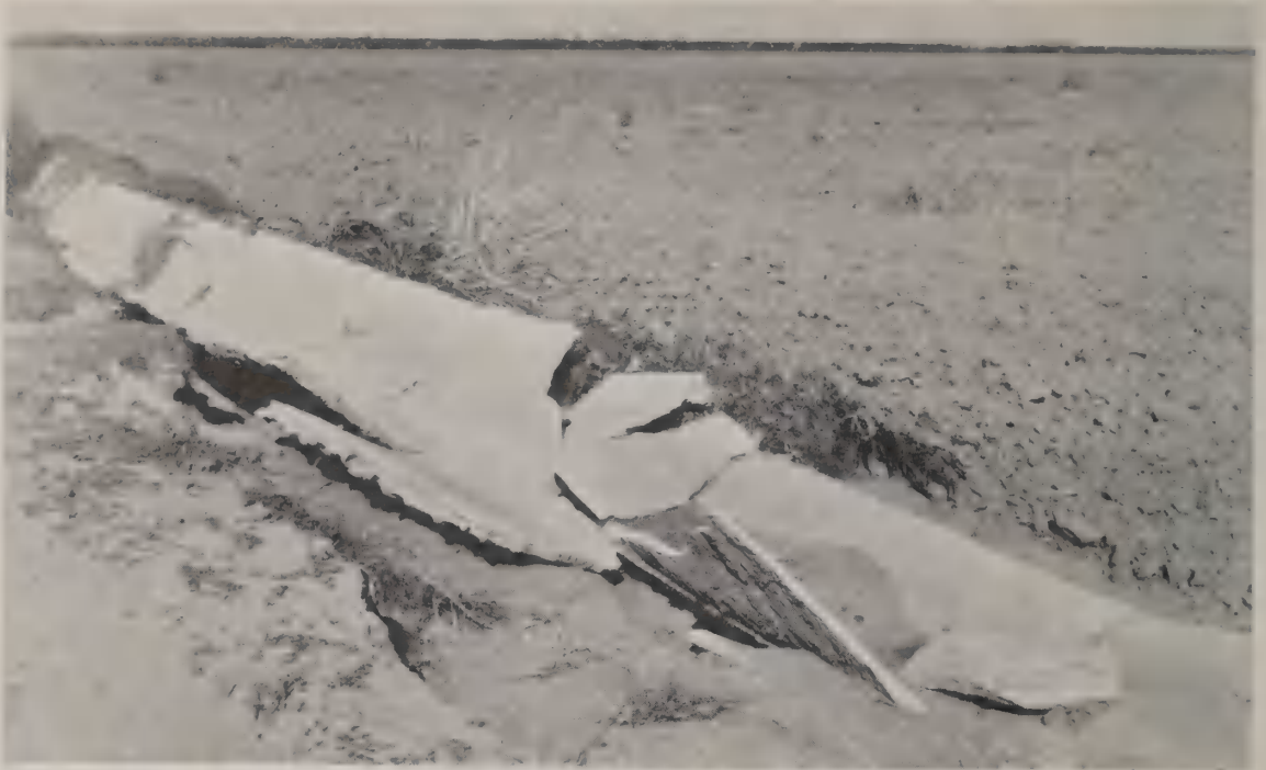
Photograph 3. Flood damage to a concrete-lined irrigation ditch (Whitewater Draw). ( SCS Photograph )
