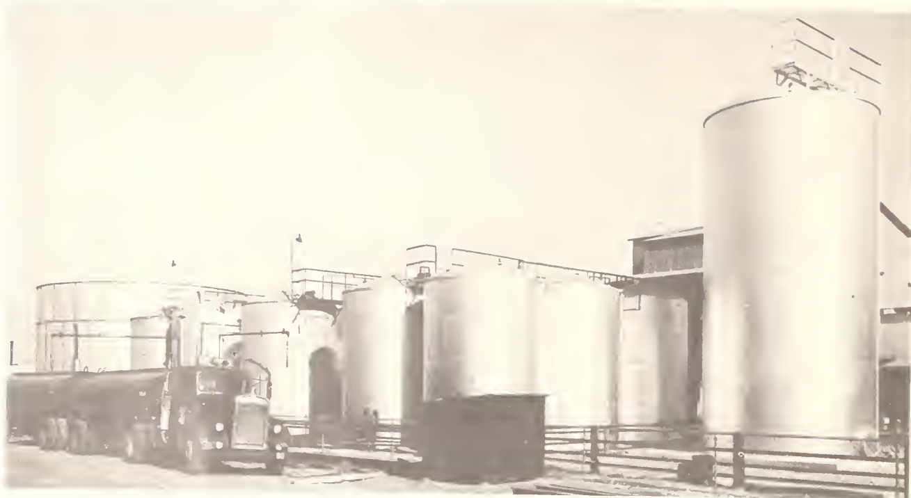
Oil-storage tanks at an oilseed processing plant.
