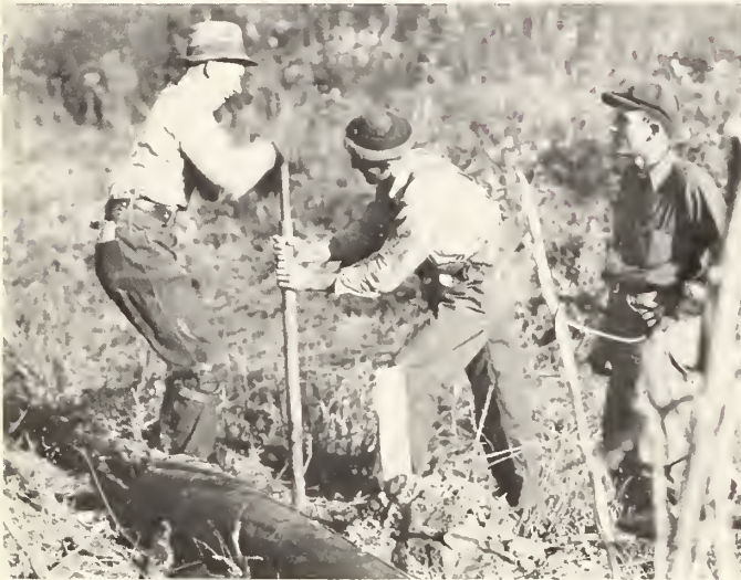
Early crews had few power tools to work with. Holes were dug by hand...
