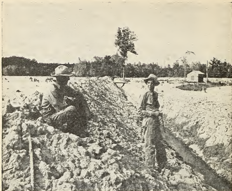
Figure 128. Much level and low-lying land in the humid parts of the United States requires drainage before it can be used for agricultural production. (U. S. D. A.)
