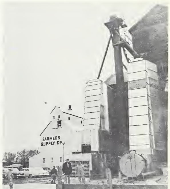
A twin drier installation. Elevators sometimes find that their original drier is too small for their needs and then install a second one to increase capacity. If possible, elevators should try to install a drier that will be adequate for future needs. For a drier with larger capacity is more economical to own and operate than two smaller driers with the same combined capacity.
