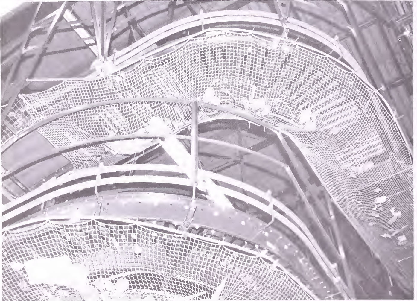
Figure 8.—Installation of nets at elevated conveyor turns to catch errant products (viewed from below).
