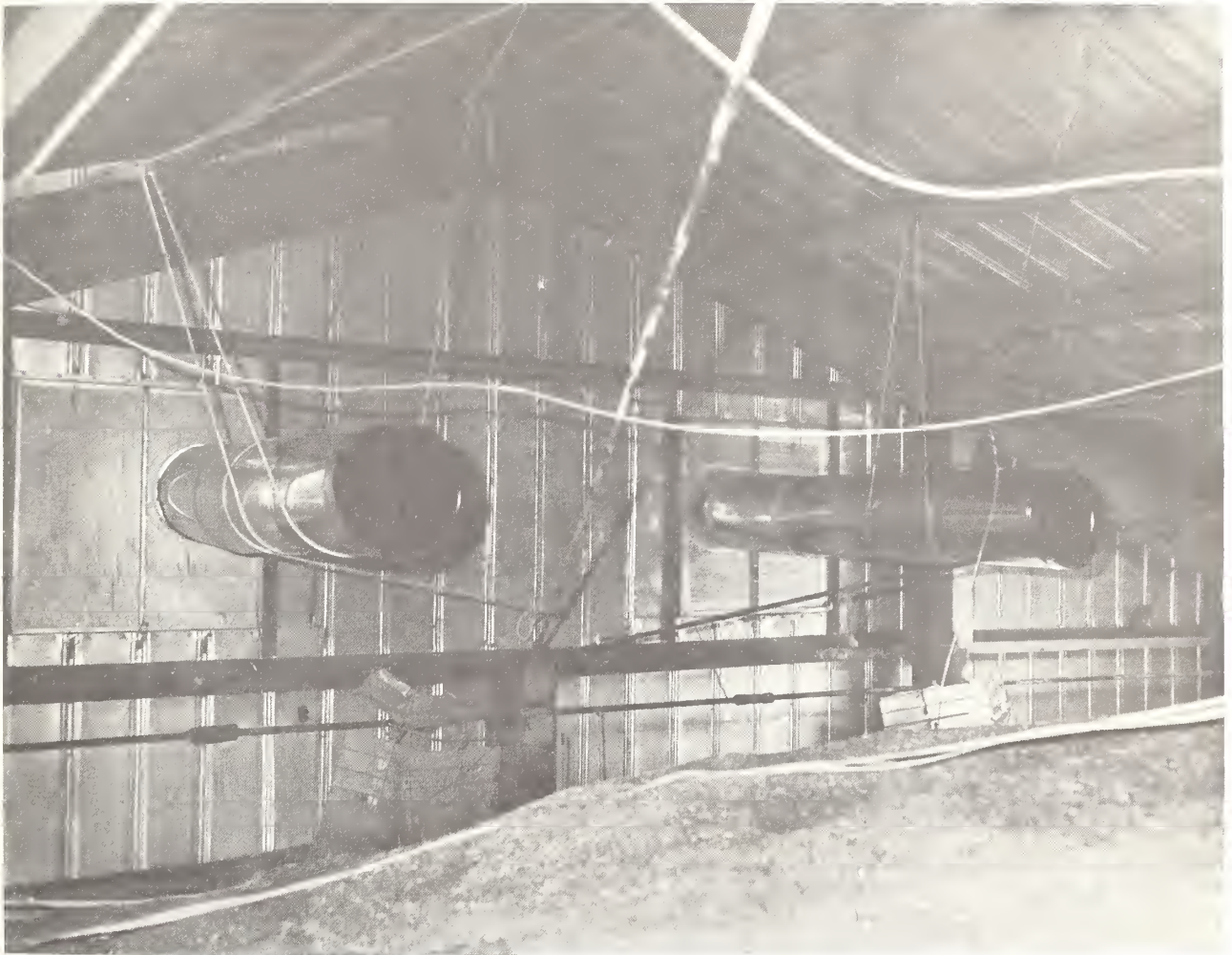
FIGURE 5.—View of the return ducts from inside a Butler building at Woodston, Kans.
