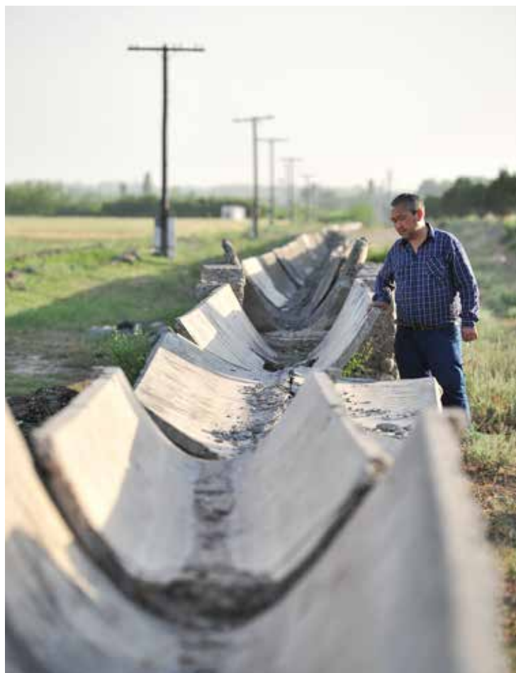
FIGURE 1. The irrigation systems of Tajikistan fell into serious disrepair after the collapse of the Soviet Union and the country's ensuing civil war (photo: Neil Palmer/IWMI).
