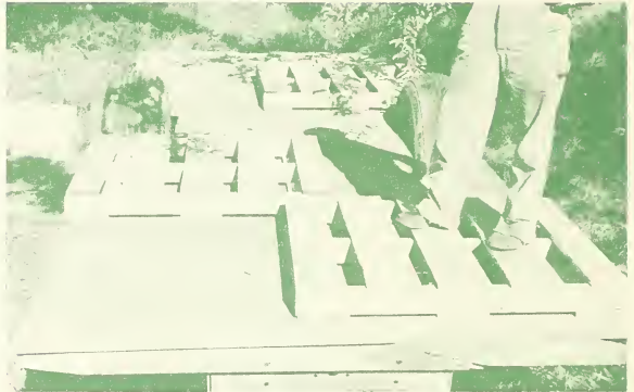
FIGURE 12. --Pallets placed on bed of trailer in preparation of partially palletized load (method D).
