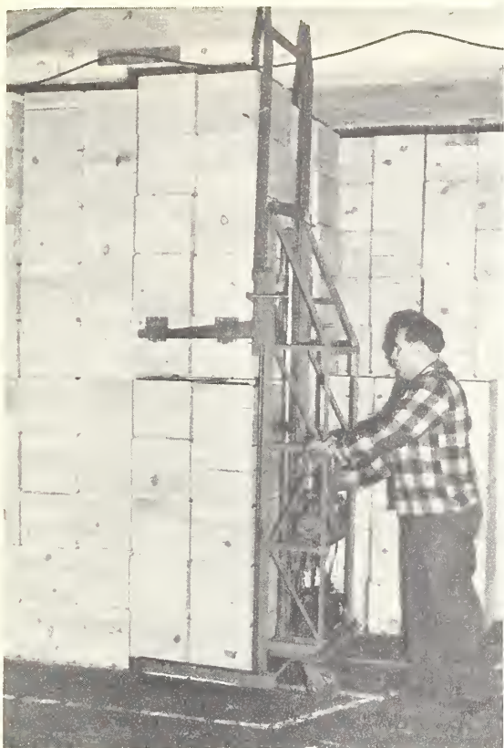
Figure 38.--A worker pushes the load forward until the top stacks are over the lower stacks. The worker then operates the hydraulic lever which lowers the top stacks into position.
