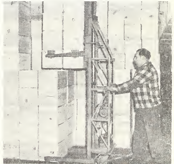
Figure 94.--The load being pulled free from the two bottom stacks. After this the stacks are lowered to the floor.
