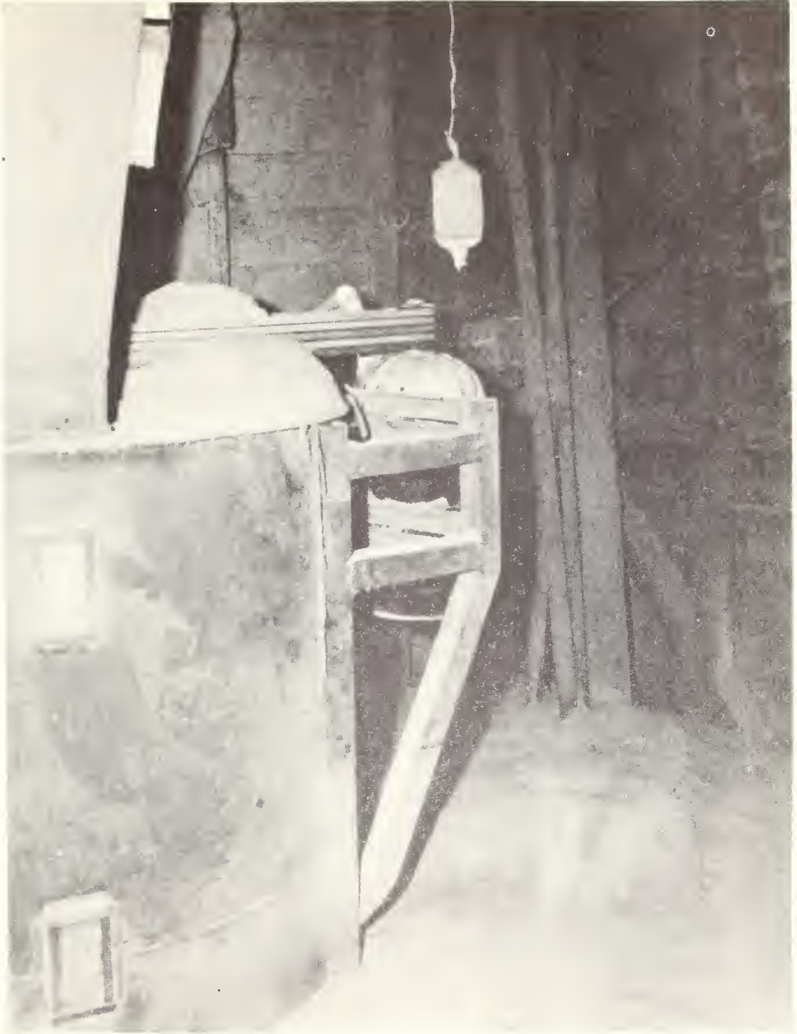
Figure 25.--Accumulation of elevator dust increases fire hazards and increases costs of operation. Here, the dust on the floor was approximately a foot deep, and the belt ran through a pile of dust which had accumulated adjacent to the motor. Any friction or electric spark is an excellent medium for expanding into a major fire. This fire hazard was located on the second floor of the elevator where visits by personnel were not frequent.
