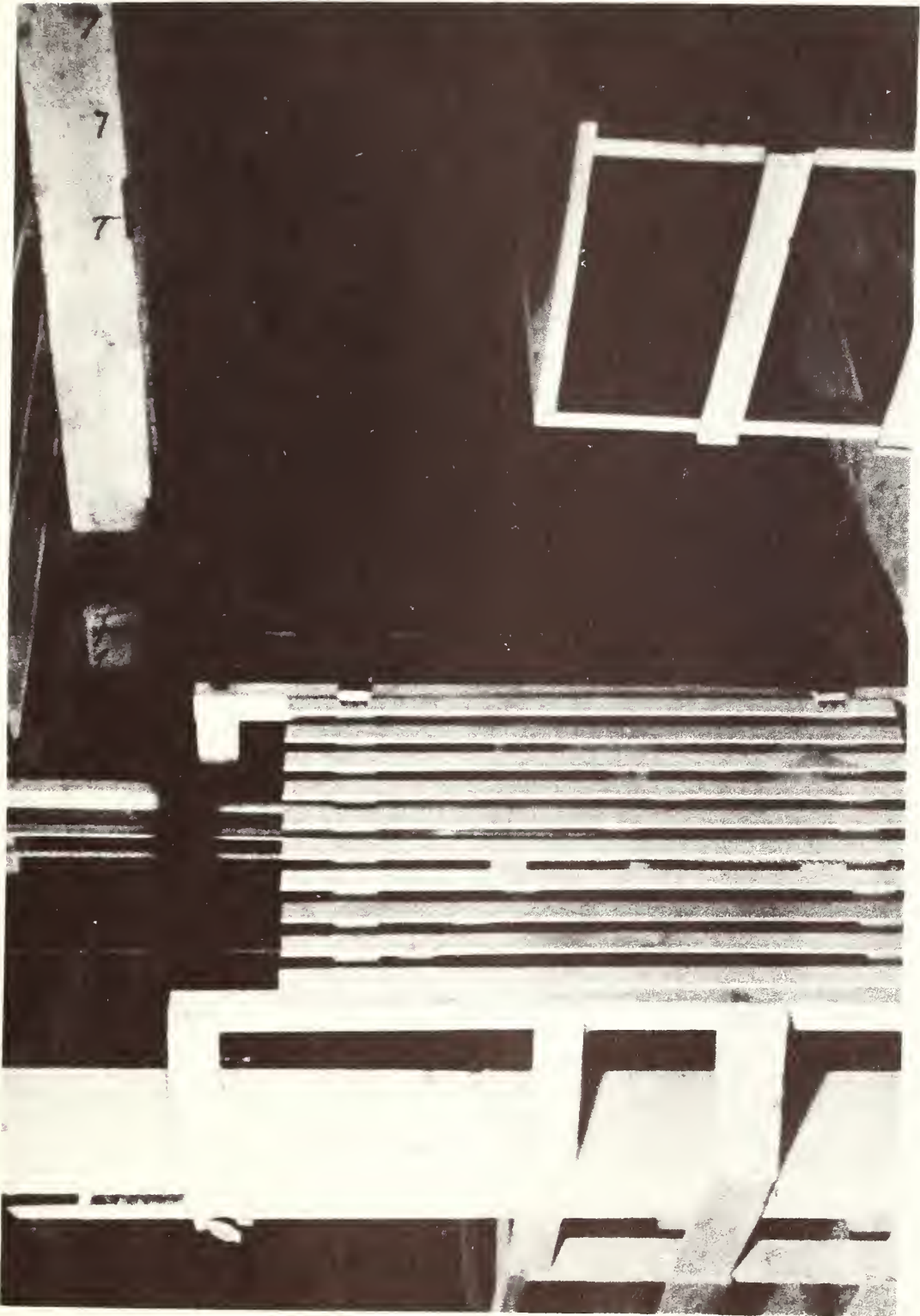
Figure 26.--Safety gates and guard rails for manlift shafts and stairway wells contribute to safety at small cost.
