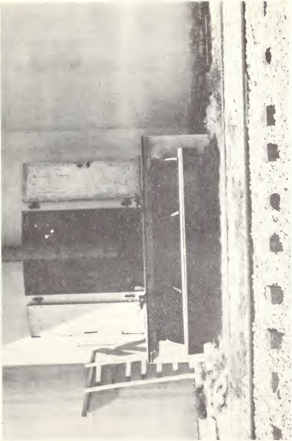
Figure 17.--A rail car grain dump, located along the spur track (underneath platform), into which grain flows from car door directly into dump pit at lower level. This device is good labor-saving equipment for elevators receiving bulk grain shipments by rail.
