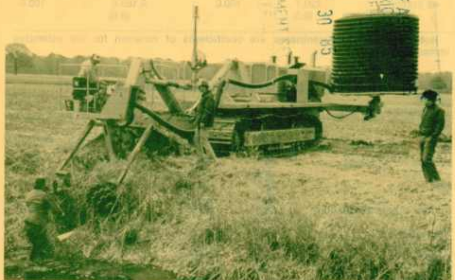
Current technology in underground drainage includes plastic tubing installed with a laser controlled mole plow. Photo courtesy of R. Wayne Skaggs, North Carolina University.
