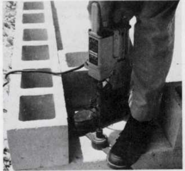
Figure 4.—Drilling to install expansion bolts. Preliminary placement of the first course of blocks without bedding them in mortar enables the builder to accurately position bolts in the centers of block cores. A bubble mounted on the drill to aid in drilling the holes vertically may be used in place of the drilling guide shown. The guide cannot be used if the first course of blocks has already been bedded in mortar.
