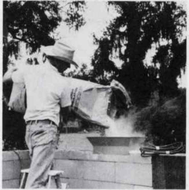
Figure 19.—Filling cores of concrete block wall with pellet insulation. Rectangular metal funnel made to fit the width of the wall reduces the filling time and avoids spillage.
