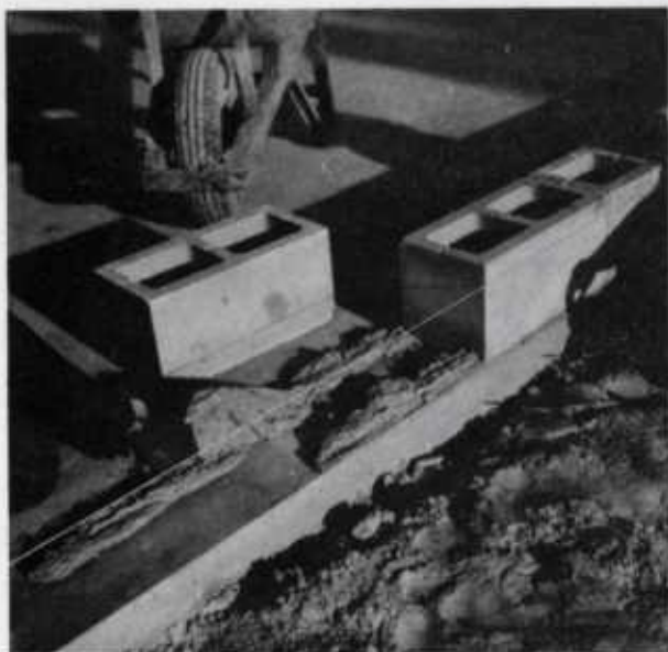
Figure 6.—Lay the first course of blocks in rich mortar on the slab floor or footing.
