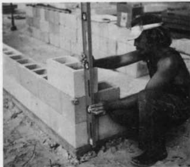
Figure 7.—Stack blocks at corners three courses high and plumb with mason's or carpenter's level.
