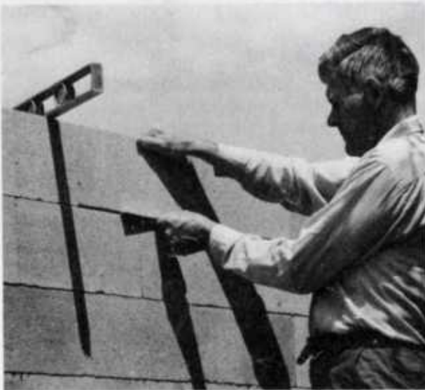
Figure 9.—Insert metal shims between blocks if necessary to level or plumb the wall.
