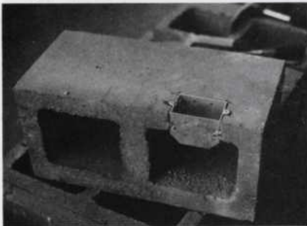
Figure 17.—Electrical outlet box mounted in sawed opening in concrete block. Box is fastened into block with 8/32 machine screws with slotted heads.
