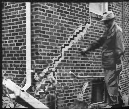
Figure 4.—Soil with a high clay content often swells when wet and shrinks when dry, thus cracking foundations unless special provisions are made during construction. This soil can expand up to 50 percent between wet and dry conditions. In addition, it may have some of the other undesirable features described elsewhere.
