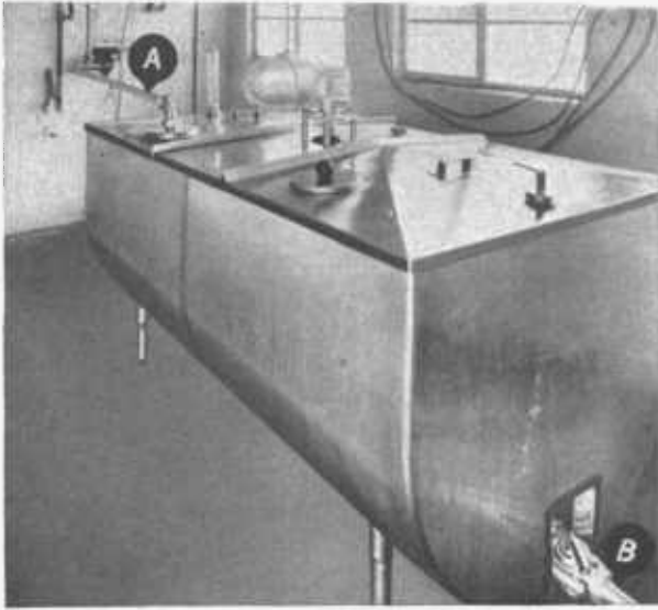
FIGURE 12.—Refrigerated bulk milk tank into which milk is piped (A) from milking room. Milk is pumped to tank truck through hose or pipe connected at B.
