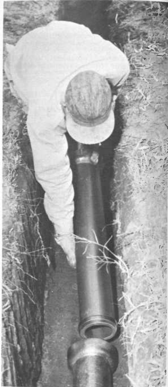
FIGURE 4.—Laying vitrified clay sewer pipe with compression-type joints of resilient materials. (Photo courtesy National Clay Pipe Manufacturers, Inc.)
