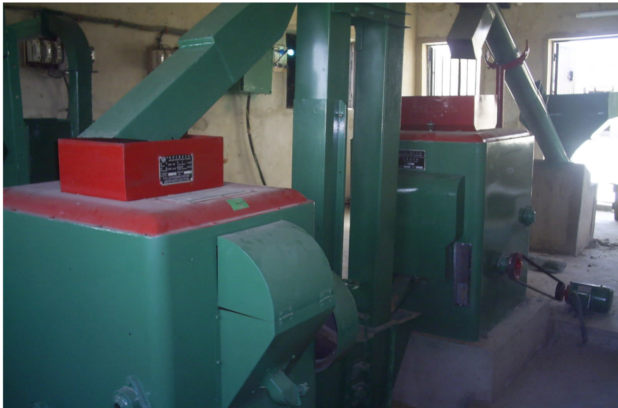
Integrated rice mill at KNAFES, Kura (note the Chinese-made primary de-stoner at rear and secondary de-stoner in front)
