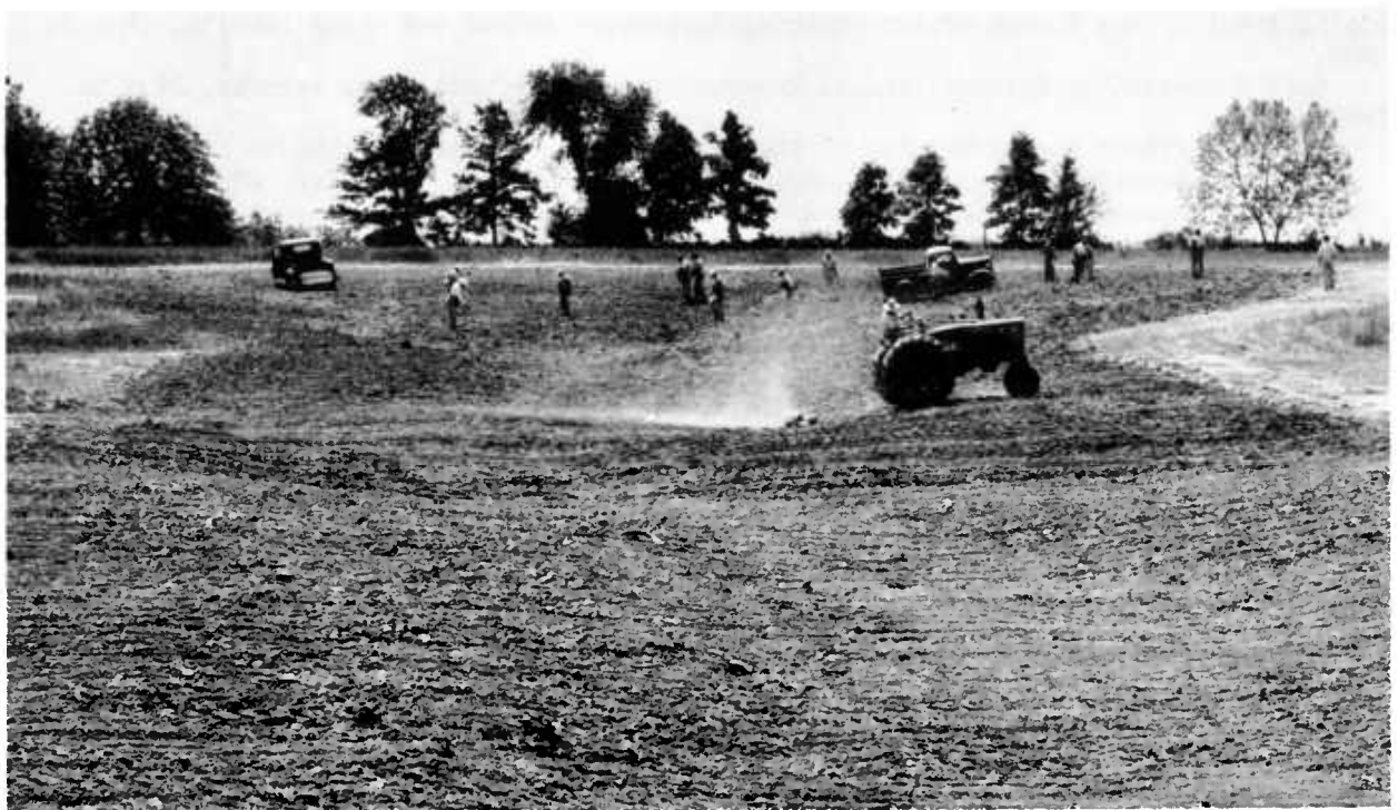
SCS Ark-61-487 A & B Figure 8.--Above, gully near Berryville, Ark., before rehabilitation. Below, gully leveled and filled, ready for sodding.
