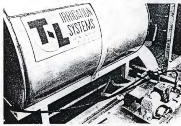
Figure 6.—Piston-type chemical injection pump and tank
