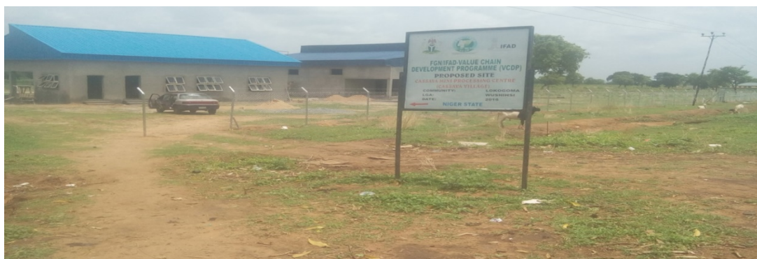
Figure 2. On-going Building by FGN/IFAD Value Chain Programme in Lokogoma Village in Wushishi Local Area, 2017
