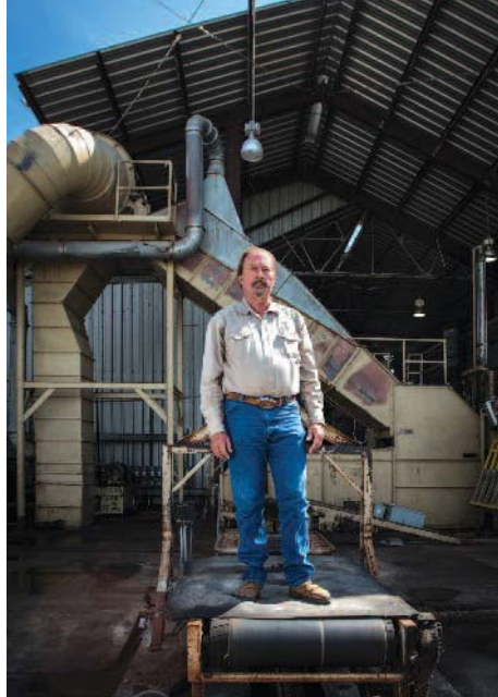
David Wyatt, manager of Bayside-Richardson Co-op Gin, stands on what is left of the seriously damaged gin in Woodsboro, Texas. Members were harvesting a bumper crop when Hurricane Harvey pounded the area, leaving multiple buildings and equipment at the gin damaged beyond repair. USDA photo by Lance Cheung
