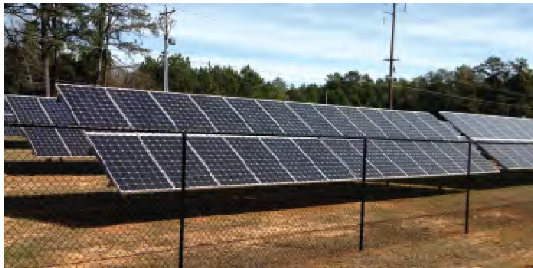
This Flint Energies solar panel array will be dwarfed by a new, 131-megawatt solar power project being constructed outside Butler, Ga. It will cover an area the size of 826 football fields. The power will be shared by three co-ops: Cobb EMC, Sawnee EMC and Flint Energies EMC.
