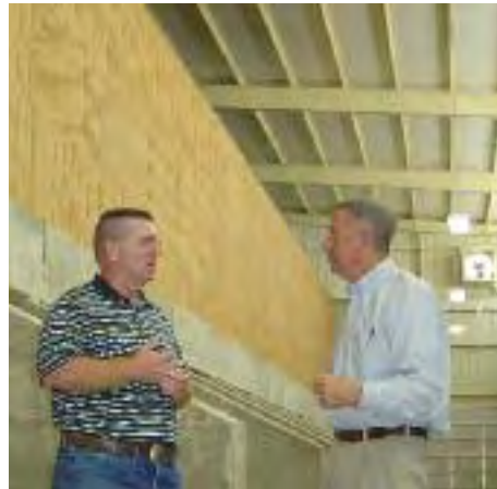
Co-op President James Deatherage, right, checks out the progress on the co-op’s new agronomy center, slated to open by fall.
