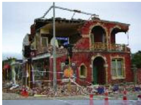
The Piko Wholefoods Co-op store sustained heavy damage in the earthquake that hit Christchurch, N.Z. The top floor of the 106-year-old building had to be demolished.
