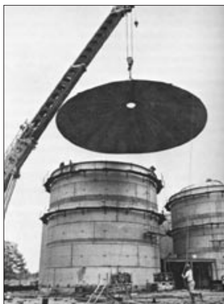
A tank lid seems to float over one of three, 700,000-gallon grape juice storage tanks being constructed for Welch Foods in Pennsylvania prior to the 1983 season.
