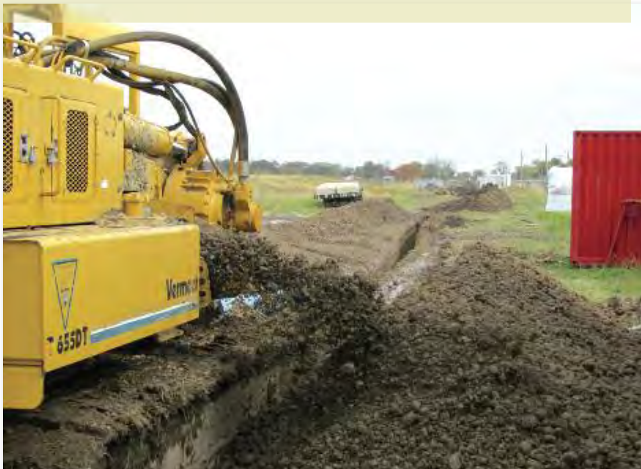
New water lines are extended to homes that are part of the EJ Water Cooperative in southern Illinois. Photo courtesy EJ Water Co-op
