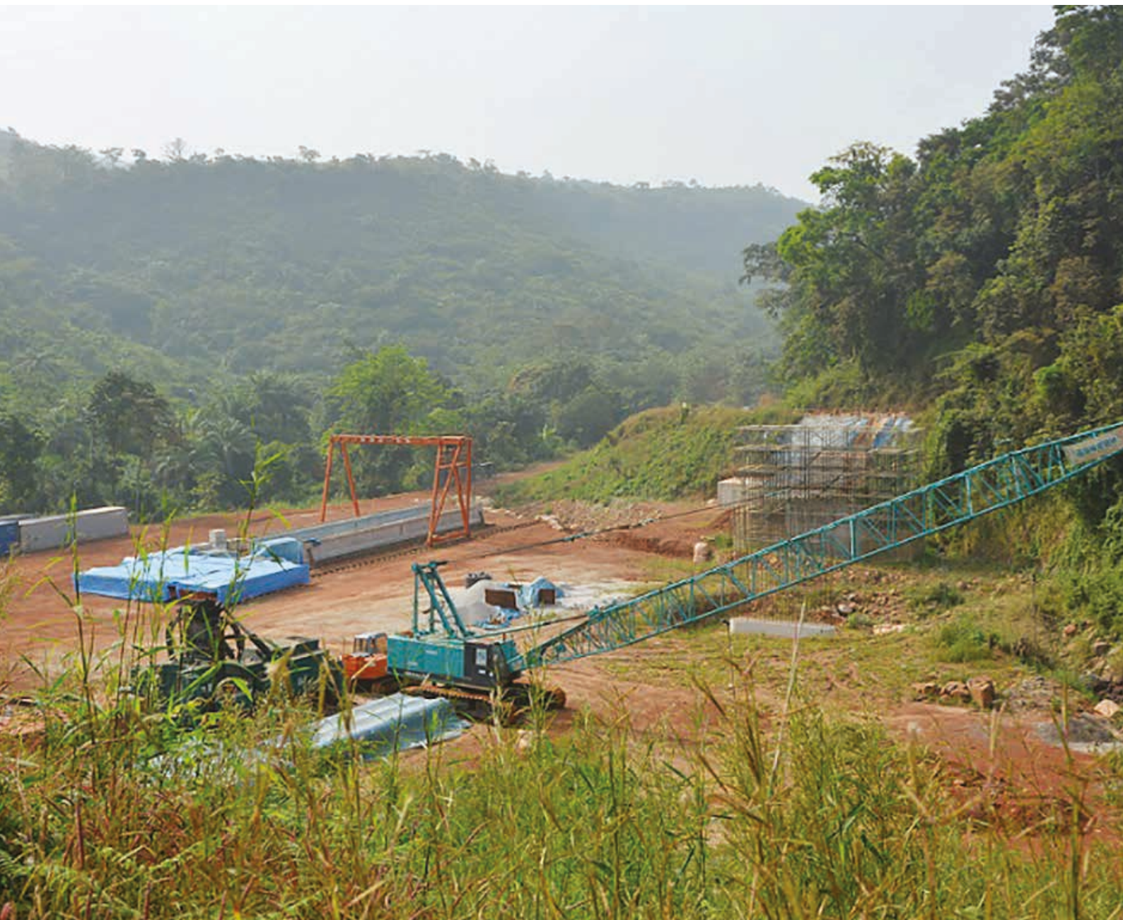
The construction site of the Kaka bridge (in the Coyah District) was stopped and abandoned by DAI Nippon Constructing, who also repatriated workers due to Ebola. Photo by UN RCO Guinea/Communication Office
