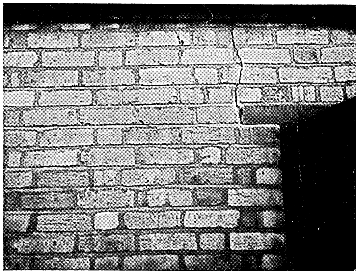
Plate 21: Mortars are sometimes stronger than the bricks they join.
