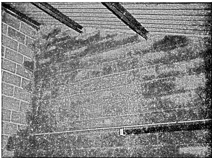
Plate 35: Penetration of damp through a gable wall.
