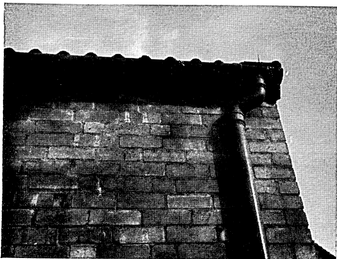
Plate 22: Poor quality mortar may shrink away from the brickwork . . . .
