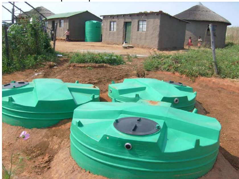
Figure 3.26: Plastic tanks (5,000 litres) installed in the Potshini catchment under a WRC funded project.
