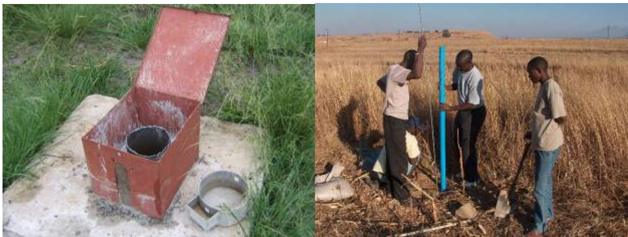
Figure 2.16: Installation of piezometers with Potshini High School pupils during their work experience week (left) and deep observation groundwater borehole (120 m deep, right).
