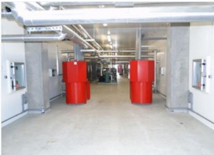
Figure 2. The interior of the ULO cold storage
